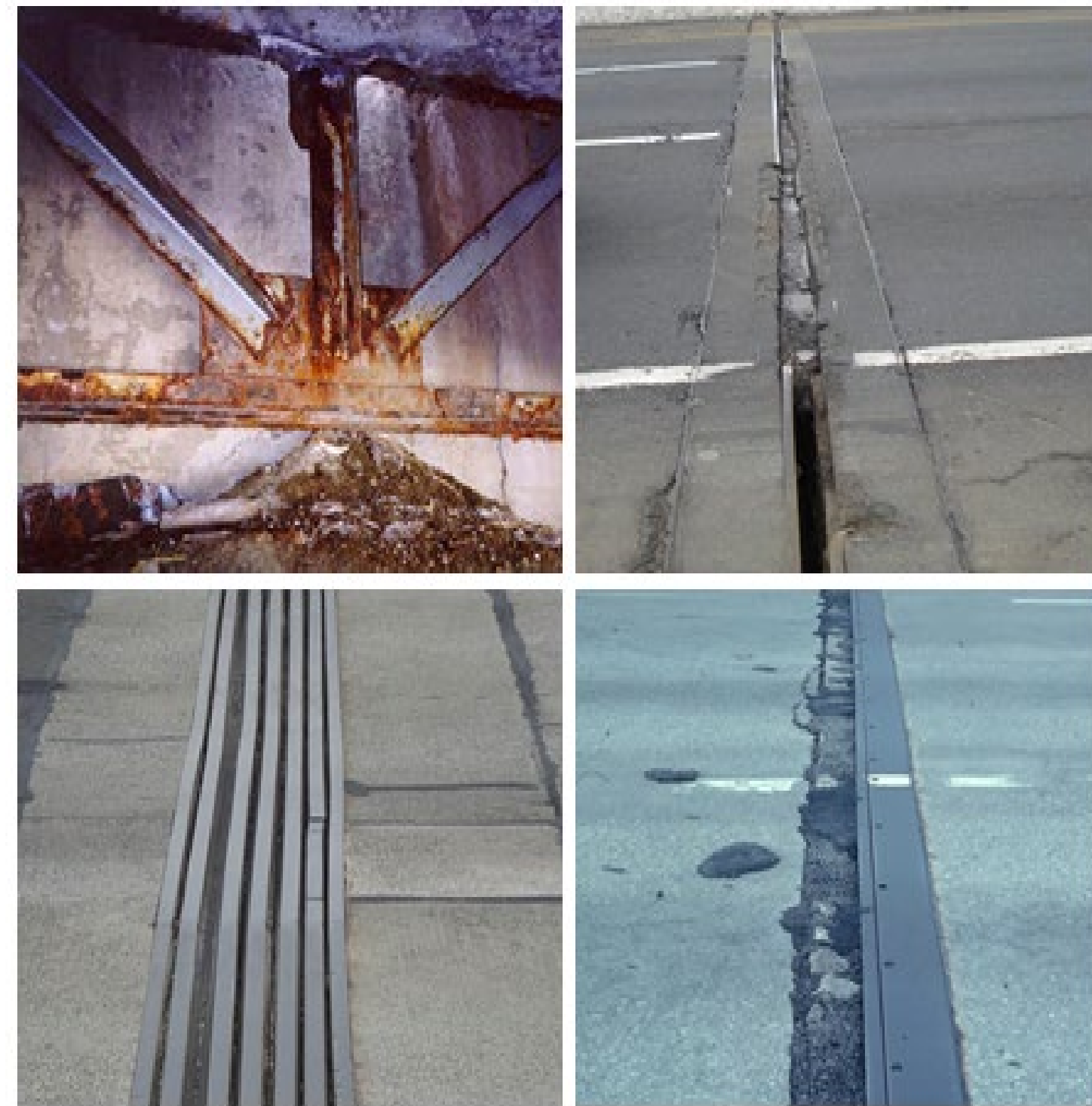
Figure 1. Damage in Expansion Joints
