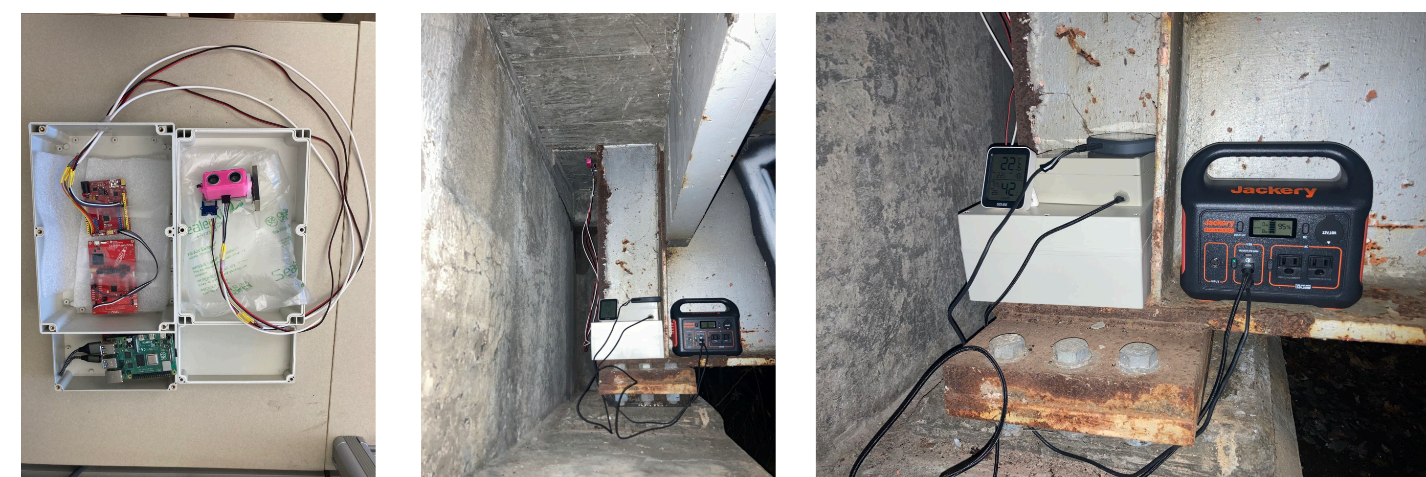
Figure 4. Deployed devices are protected by sealed enclosures
