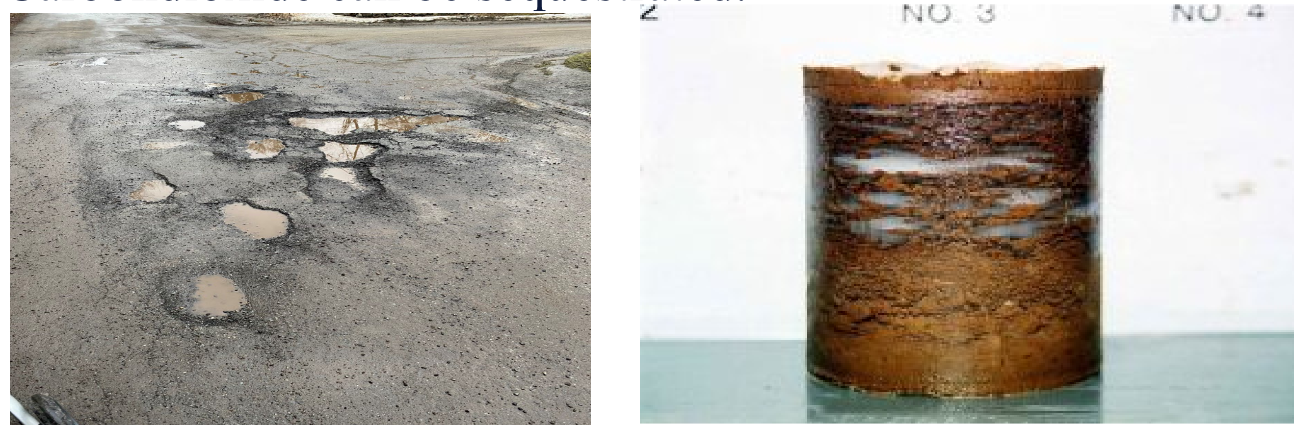
Fig 1: Failed pavement Fig 2. Freezing and thawing in pavement
