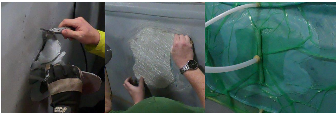
Figure 18: Repair of Structural Defect: Left: Removal of Affected Laminae, Center: Layup of New Fabric, Right: Re-Infusion
