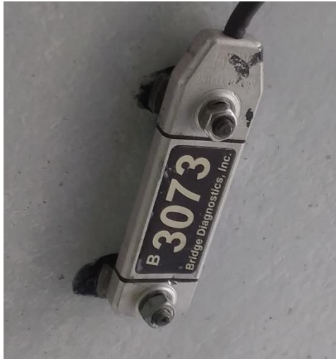
Figure 21: Strain Transducer Mounted to the Bottom Flange of a Girder
