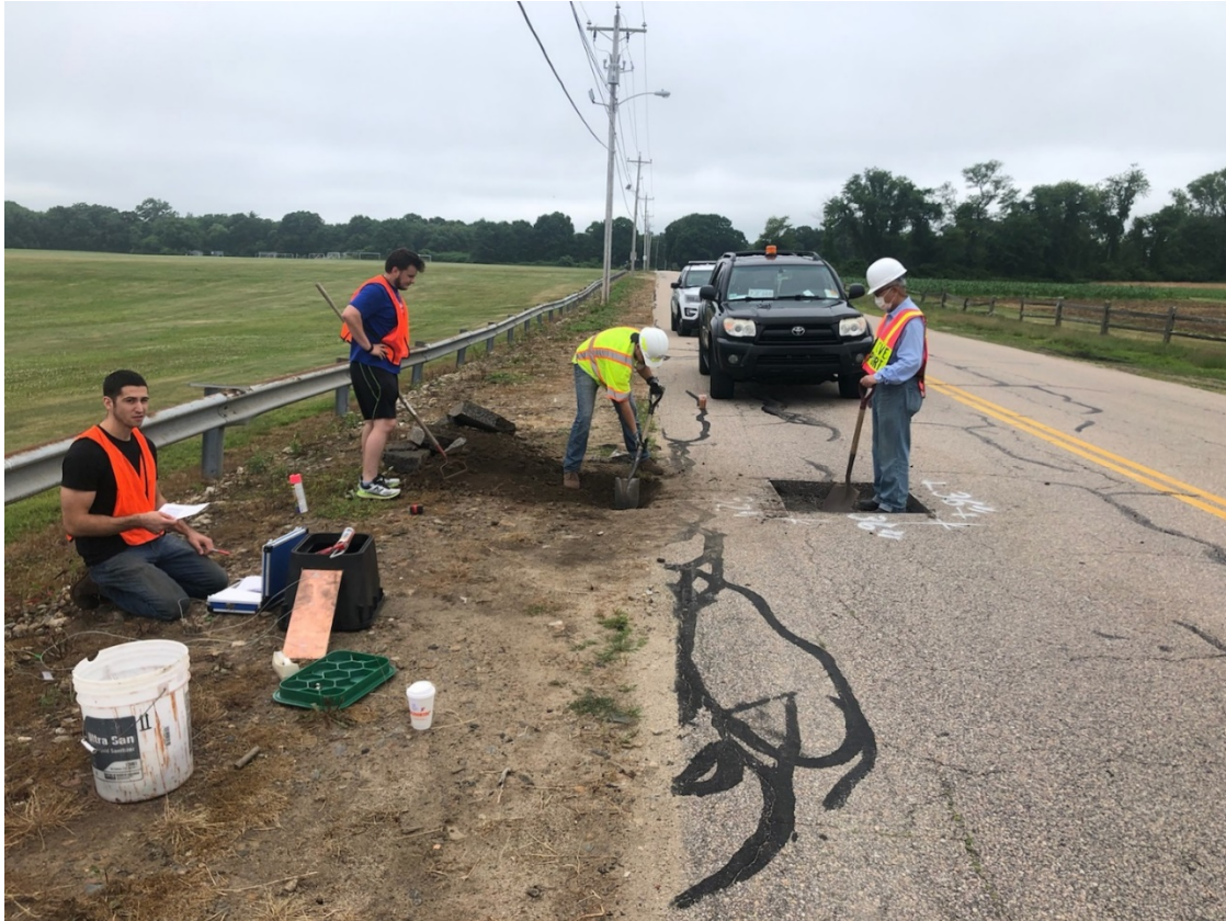
Figure 3.8. Digging a hole for the irrigation box in the shoulder of Plains Road. From left Austin DeCotis, Stephan Zaets, Kevin Lapierre (digging), K. Wayne Lee (standing where the sensor will be installed).
