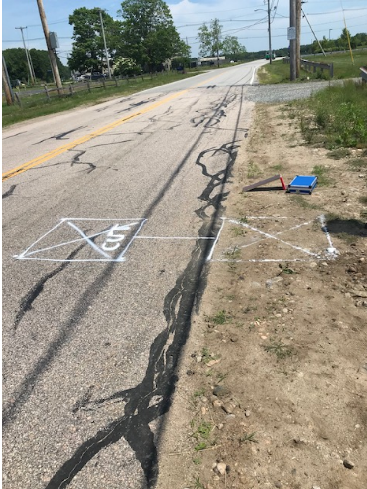
Figure 3.7. Markings for the saw cuts for strain sensor (in the road) and energy harvester (in the shoulder) on Plains Road in Kingston, RI.
