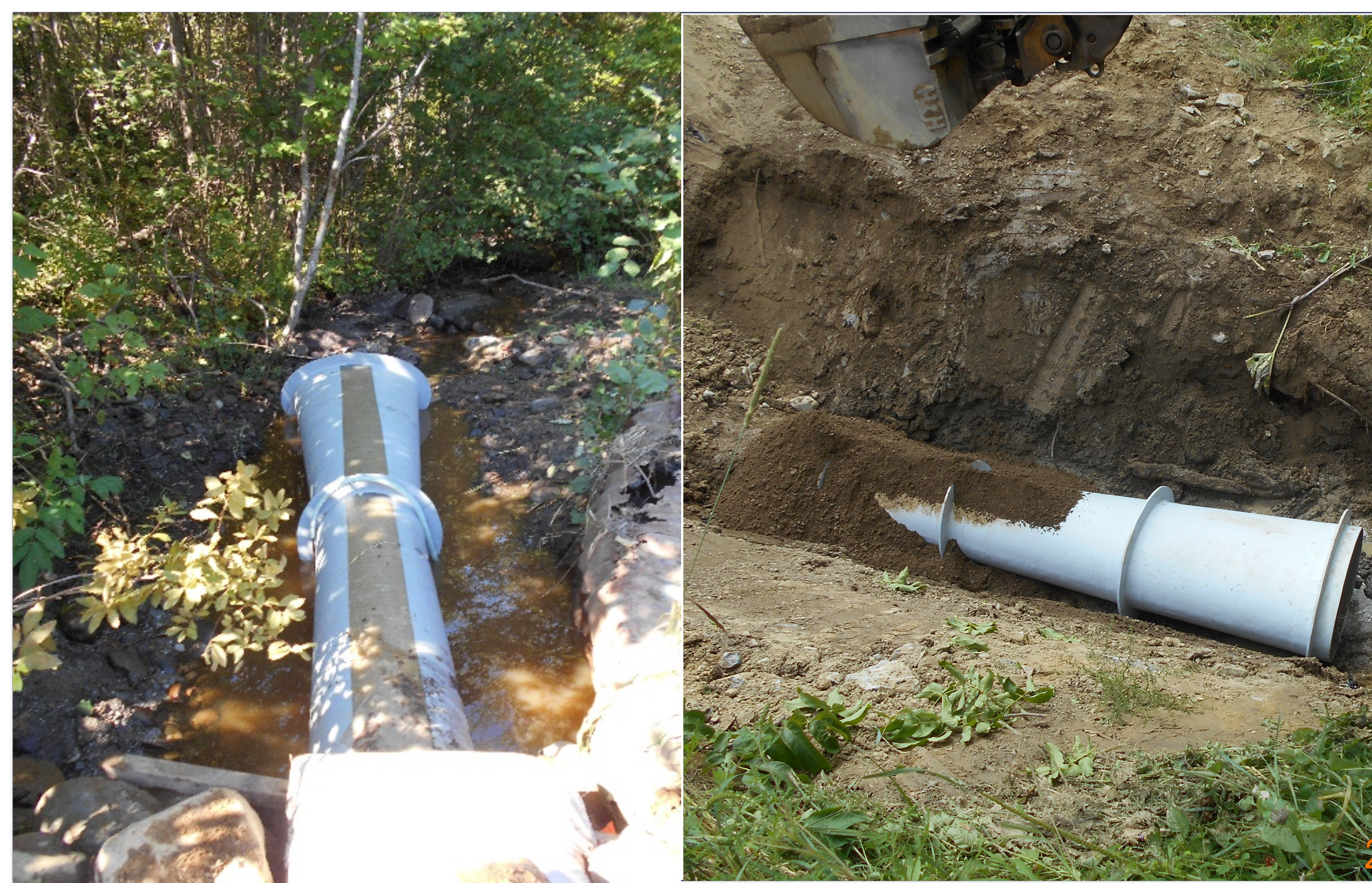
Fig: Fiberglass culvert diffusers. (courtesy-Alexandar Mann, PE, MaineDOT)
