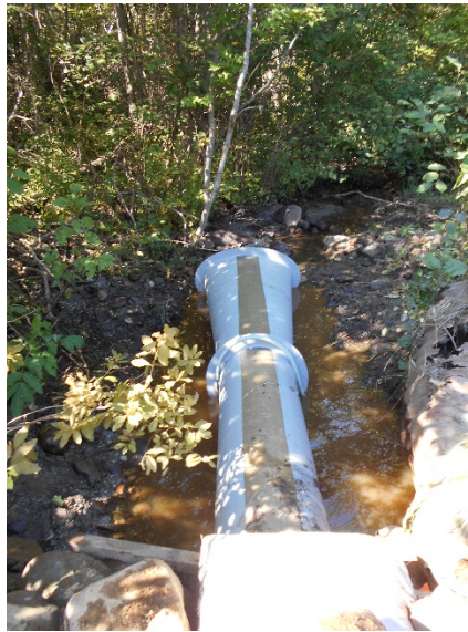
Fig: Fiberglass culvert diffuser at Thorndike Maine. (courtesy of Alexander Mann, PE, MaineDOT)
