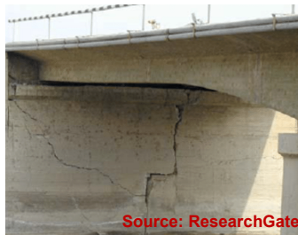
Cracks on concrete abutments
