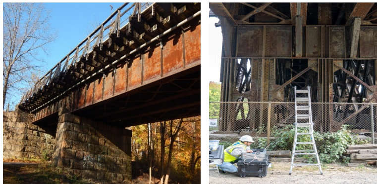
Figure 1 (A) Side view of Salmon Fall Bridge (NH). (B) UML team working on site.
